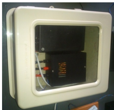
Figure 6: Controller unit inside the casing
